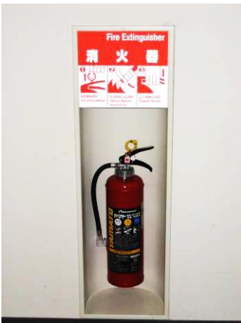
Fire extinguishers are located in hallways and some rooms
