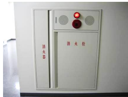
Fire alarm (top) and hydrant (bottom)
