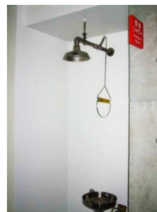
Emergency shower (wall-hanging type) : Pull the chain for a rinse. The shower will stop automatically.
